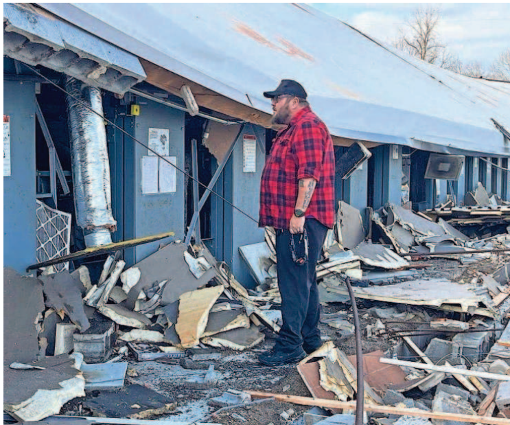
Tanner Watkins, a game technician at Big Play in Hendersonville, looks through sections of the building reduced to rubble. ANDY HUMBLER/THE TENNESSEAN
